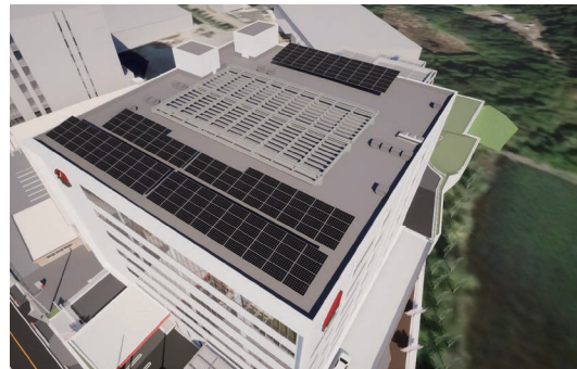
Installing solar panels at the new building of the Global Headquarters and R&D Center (*image)
